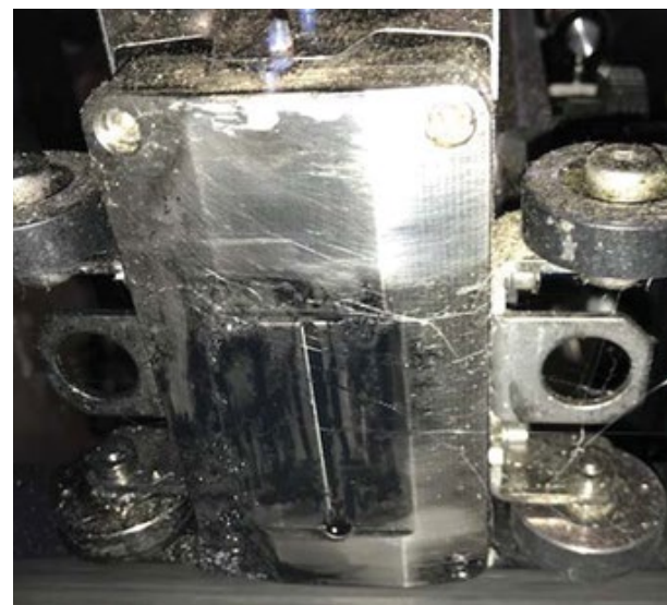
Dust and debris (hot melt glue)
